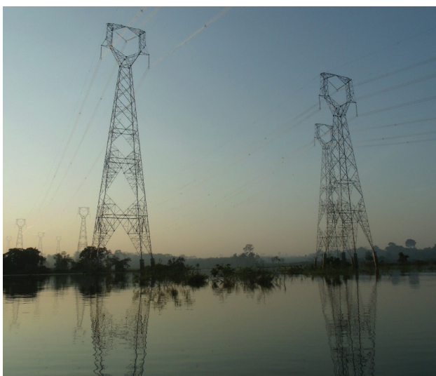
Figure 13 – Transmission line of the Santo Antônio HPP, Jaciparaná River/state of Rondônia (Photo: Aderson Alcântara).
